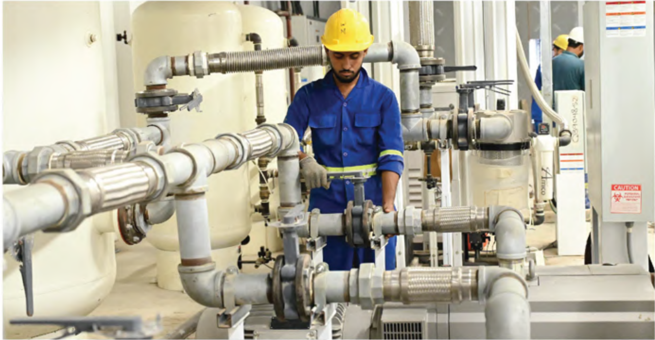
World's largest medical air plant supplied and installed by Pakistan Oxygen at a prestigious hospital in Karachi.
